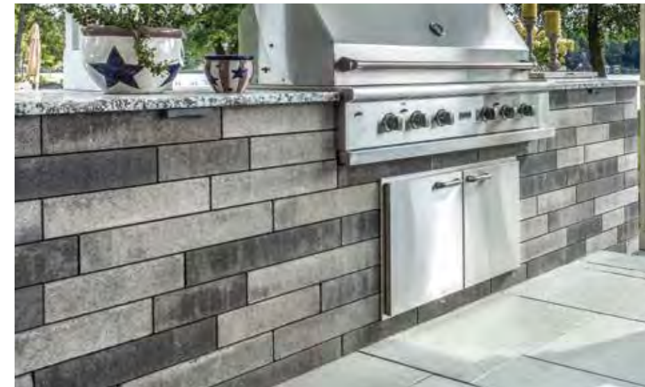
LINEO™ DIMENSIONAL STONE This modern grill island is built using Lineo Dimensional Stone (page 110).
